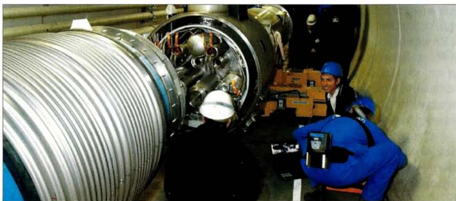
The 128th CERN Council meeting heard about installation plans for the LHC. Tests on installing magnets in the LHC tunnel were carried out earlier this year.
