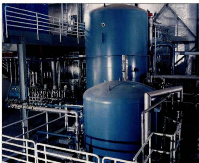
The 2 and 4 K cold boxes inside the Central Helium Liquefier for the CEBAF facility at Jefferson Lab. (Photo: Jefferson Lab.)
